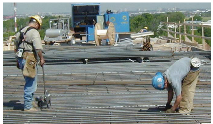
Figure 1: Rebar tying using a rebar tying machine (left) and manual tying using pliers (right).
